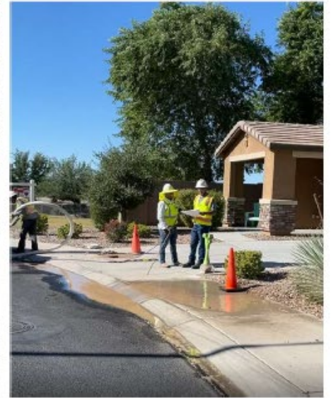
Pothole and Clean up
