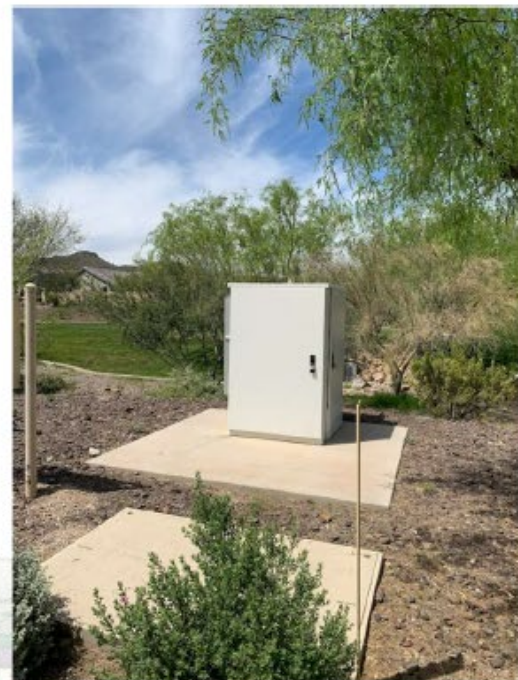
One Cabinet to Serve 10k+ homes
