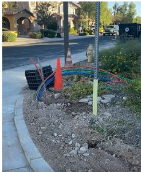
Handhole at the edge of neighborhood
