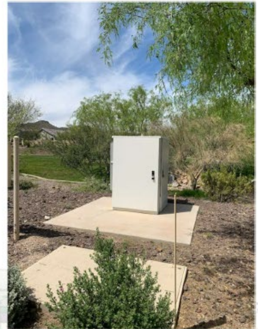
One Cabinet to Serve 10k+ homes
