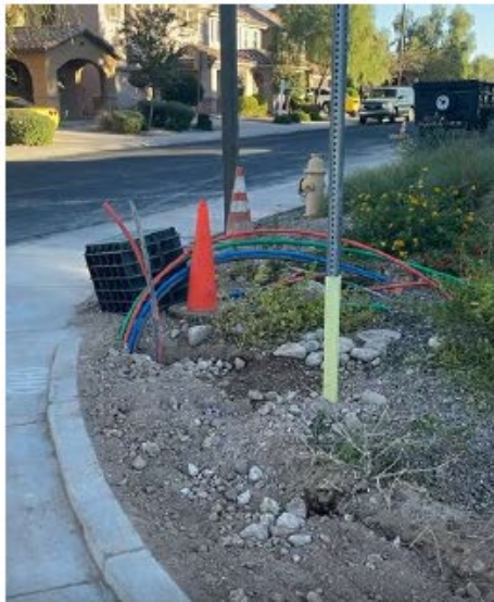
Handhole at the edge of neighborhood
