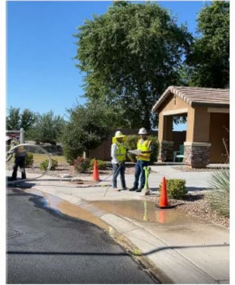
Pothole and Clean up
