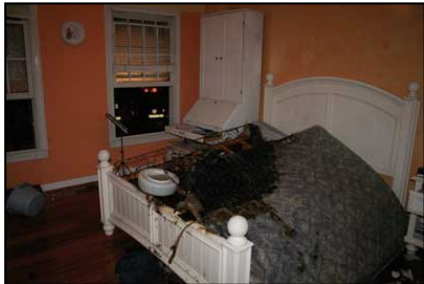
FIGURE 3-24: Bedroom Fire Extinguished by One Sprinkler
