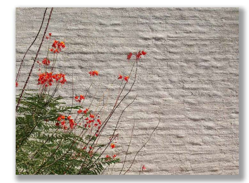
PAINTED SLUMP BLOCK W/ HEAVY MORTAR WASH
