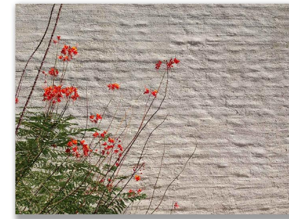
PAINTED SLUMP BLOCK W/ HEAVY MORTAR WASH
