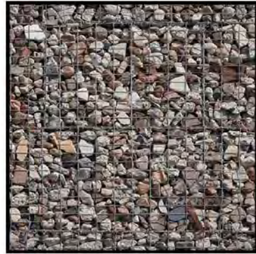
GABION WALL 6" - 8" ANGULAR RIP RAP NATURAL COLOR GABION BASKET WITH NATURAL FINISH
